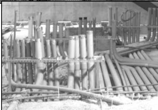
Feeder conduit for electrical room switchgear
